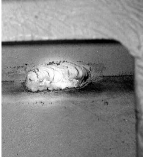
FIGURE 5.19 Cracked weld on machine housing.
