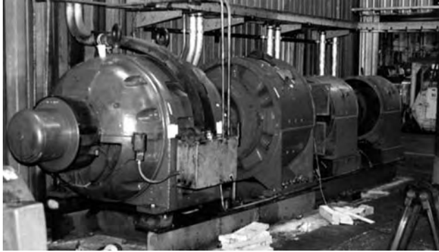
FIGURE 21.58 Typical motor–DC generator set.
