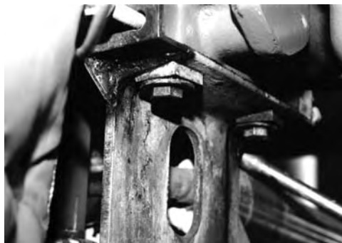
FIGURE 3.68 During a torque check on a steam turbine sway bar, the bolts threaded into the underside of the outboard bearing were found to be loose. Channel iron was used for the sway bar and the wedge-shaped washers would loosen after a short period of time from the vibration of the machine. The bolts were tightened, the vibration on the outboard bearing would be acceptable for a period of time but as the bolts began to loosen again, the vibration would steadily increase to unacceptable levels.
