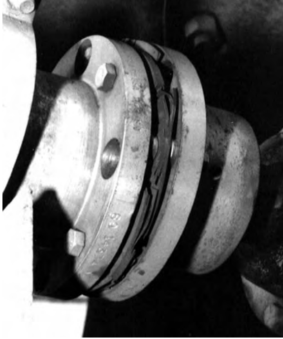
FIGURE 1.1 Disk coupling failure due to shaft misalignment.
