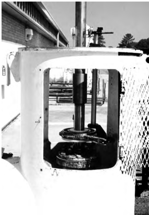
FIGURE 5.27 Measuring runout on a vertical drive shaft above a threaded coupling.
