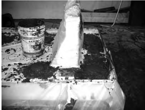
FIGURE 3.53 Grout began swelling at low end.
