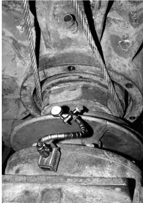
FIGURE 5.3 Performing a lift check on a pump shaft.
