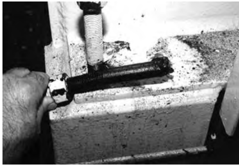
FIGURE 3.67 During a torque check on an anchor bolt, it was discovered that the anchor bolt had sheared and an attempt was made to tack weld the anchor bolt so no one would notice.
