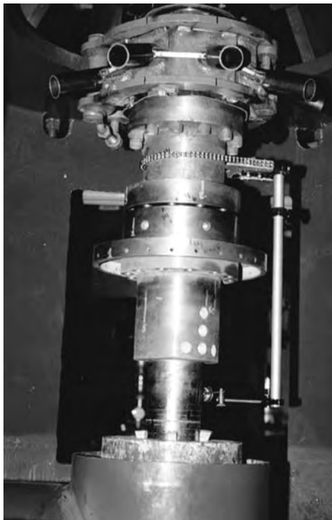
FIGURE 21.25 Alignment readings taken at the bottom of the pump shaft just above the stuffing box.
