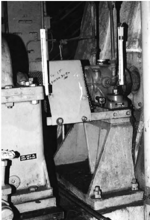
FIGURE 16.38 Scale targets mounted on gearbox and fan bearing near their centerline of rotation.
