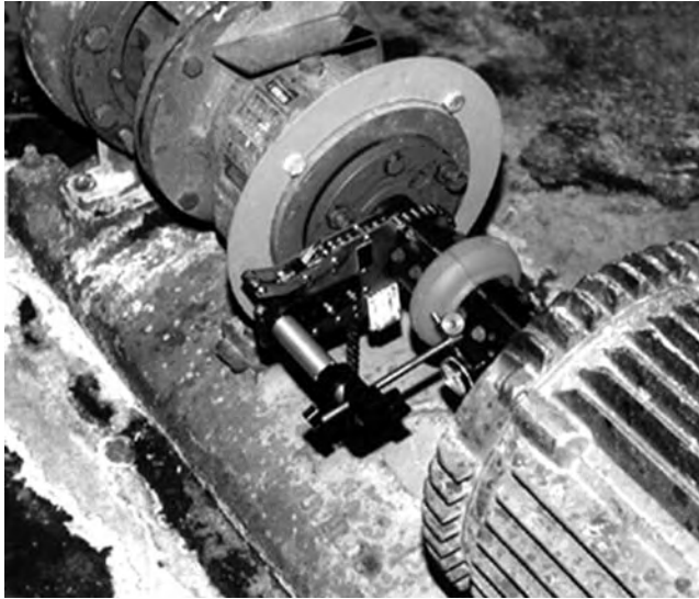
FIGURE 6.36 Pump shaft with bracket and indicator rotated 90° to side of motor shaft, stopped, and indicator reading recorded.
