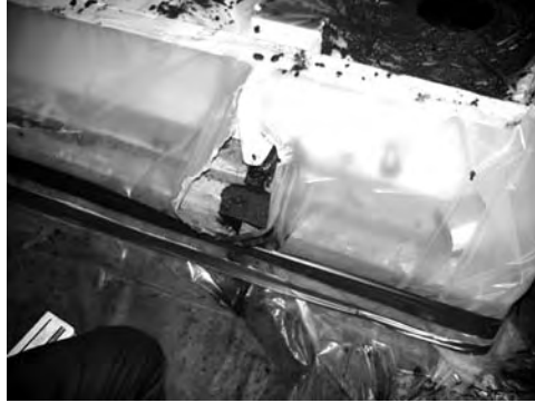
FIGURE 3.50 Grout leak around form.
