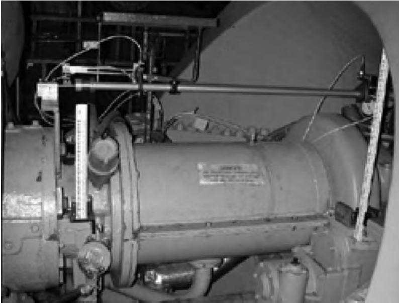
FIGURE 16.79 BRTC system measuring OL2R movement of steam turbine and pump.
