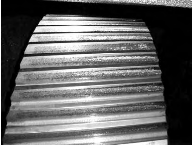
FIGURE 21.80 Irregular gear tooth wear pattern due to a soft foot condition distorting the gear housing.
