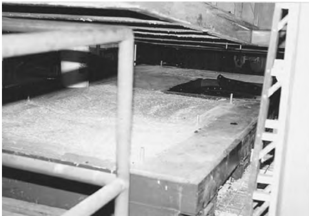
FIGURE 3.17 Inertia block for motor—fan drive. (Courtesy of Unisorb, Jackson, Michigan. With permission.)
