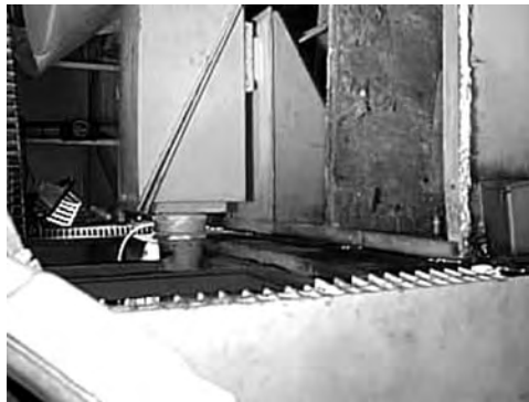
FIGURE 5.49 Soft foot correction shims for a motor.
