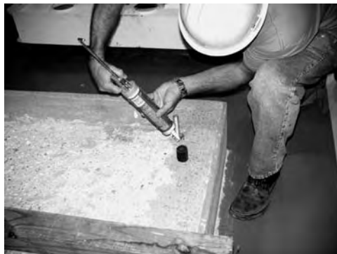
FIGURE 3.30 Sealant applied to anchor bolt to prevent grout from entering the protective sleeve.
