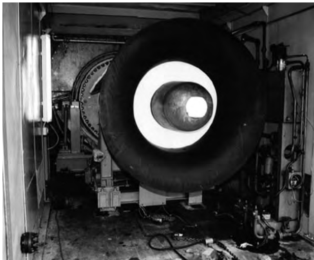
FIGURE 21.8 Gas turbine driving an electric generator.
