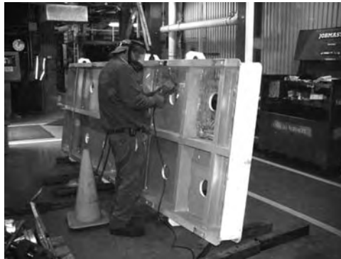
FIGURE 3.29 Paint on underside of baseplate removed to insure good bonding with epoxy.
