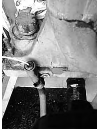
FIGURE 5.51 Soft foot correction shims for a pillow block bearing on a fan.
