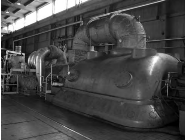
FIGURE 21.6 Large steam turbine.
