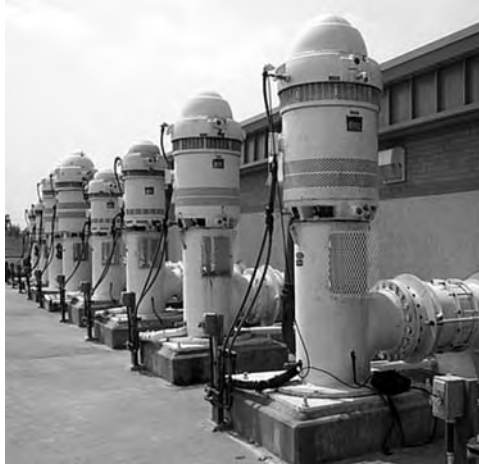
FIGURE 21.17 Medium-sized vertical pumps.
