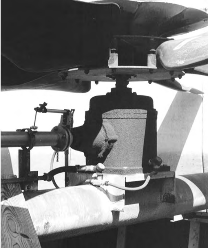
FIGURE 13.3 Shaft to coupling spool method used on cooling tower fan drive with bracket attached to gear input shaft and indicator taking reading on spool.
