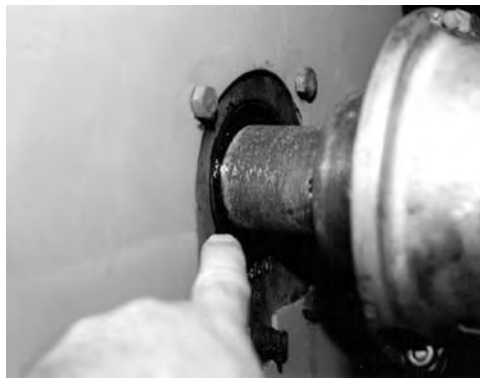
FIGURE 5.18 Oil seal installed backwards on a motor.
