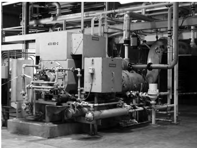
FIGURE 21.3 Large electric motor supported in sliding bearings.
