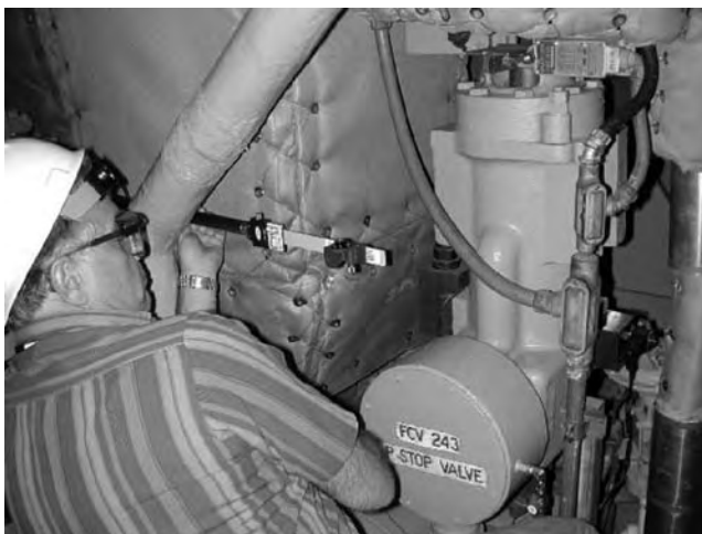
FIGURE 16.49 Jig transit and scale target on outboard pump bearing for lateral measurement.
