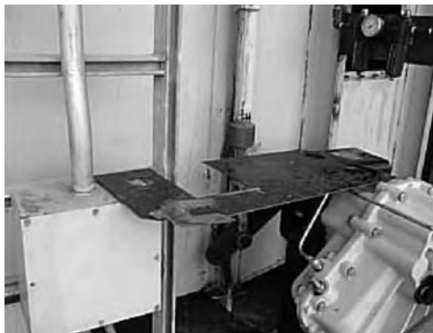
FIGURE 5.36 Shim pack that had worked loose under a fan bearing due to a soft foot condition.
